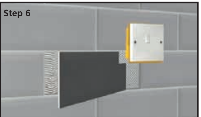
Step 6 Tile with a clean edge to work from. The Safety Shield also ensures sufficient space is left to recess the fitting.
