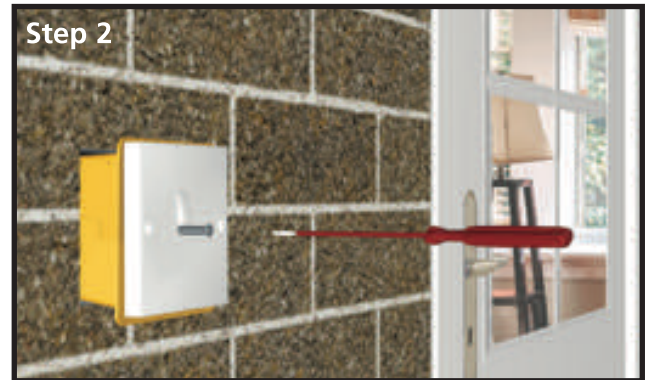
Step 2 Second fix - Insert the Safety Shield into the back box, refix the electrical fitting and complete safety tests.
