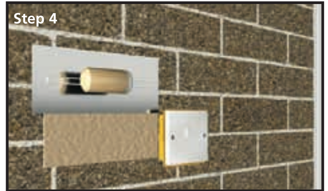
Step 4 Plaster, allowing a clean edge and prevent excess moisture and plaster entering the electrical fixing.
