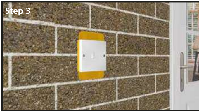
Step 3 The electrical supply is safely maintained during the remaining building work and the electrician can leave site.
